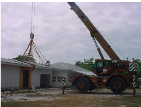
Works being carried out for the Community Resource Centre at Cocos (Keeling) Island
